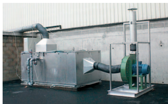
Panel 6: The SORBICAT pilot plant
