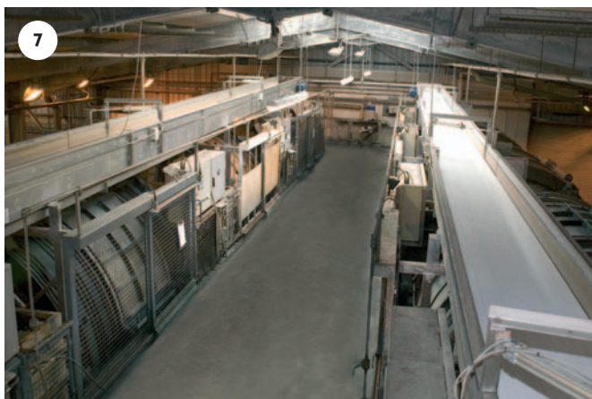
Figure 7: Delivery conveyors with diverters run above tan drums
