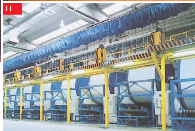
Figure 9: A five drum installation with loading and unloading conveyors (Baggio)
