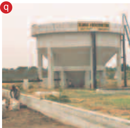
Typical large scale sludge thickening plant.
