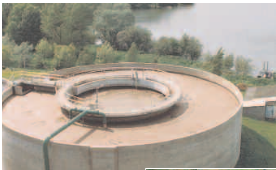
As part of nitrogen removal, the anaerobic section can be constructed within the aerobic part. Stirrers keep the effluent in motion within this central section.
