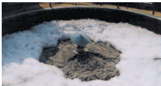
After anoxic treatment the effluents need degassification to oxidise and flush sulfides from solution of effluent, before offer to the activated sludge treatment stage.
