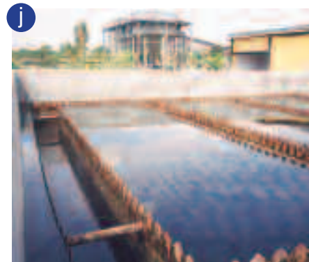
Tertiary settling after chemical dosing. The clear supernatant flowing over the notched weir is ready for discharge as treated effluent.
