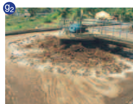
g 2 Surface aerators are most commonly used for mixing and aeration.
