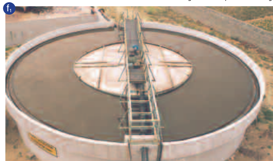
The chemically dosed effluent is delivered to the centre area of the clarifier, and directed towards the tank base to assist settling. The 'bridge' spanning the tank is part of a slow-moving scraper mechanism.
