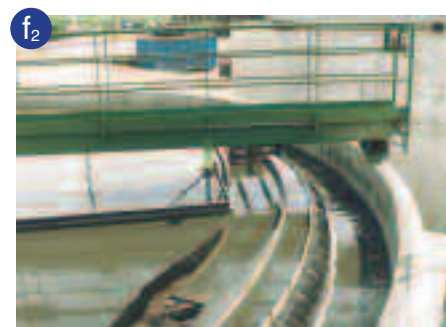
Image shows weiring of the clarified effluent, and details of the roller arrangement supporting the scraper mechanism.
