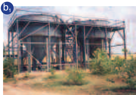
These massive primary settling vessels are carefully designed so that the settled solids can flow as a sludge from the conical base without danger of blockage.
