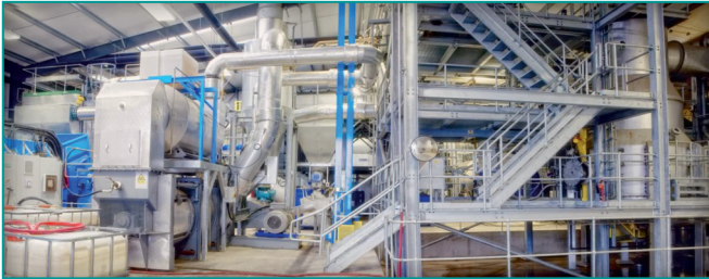
The waste-to-energy plant that Scottish Leather Group developed at the group's Bridge of Weir facility. This led to an "industrial epiphany" that there are circular ways to make high-quality leather.
