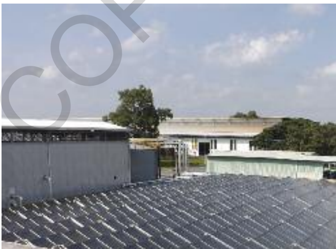
365 solar cells, covering an area of 5,400 square metres provide 1,800 tonnes of hot water (at 85°C) per day. The water is used for processing and wastewater sludge drying.
