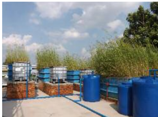
Pilot scale reed bed with a capacity to treat 3,600 cubic-metres is being investigated for end of pipe effluent polishing.
