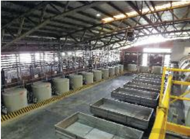
20 Hüni automated dosing polypropylene drums allow for safe and efficient chemical dosing to the retanning and dyeing drums. These drums hold the most commonly used liquid chemicals.
