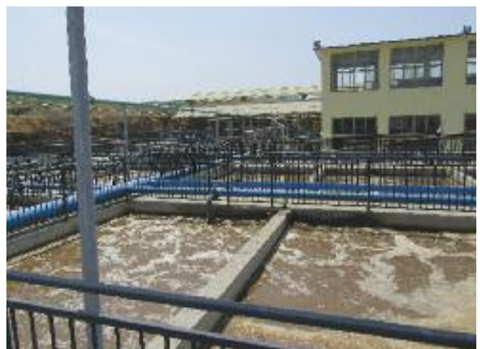
Biological treatment of the vast wastewater effluent treatment plant. These tanks constructed above ground are 15ft tall. The building in the background with the open roof is where filter cake is stored to further dry before sending off site for treatment.
