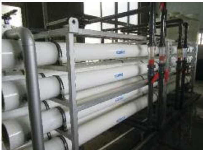
One of the two sets of membranes used for the end of pipe effluent treatment. The sight glasses show the clarity of the treated water. Prior to discharge, the treated wastewater is automatically sampled and tested by the local authorities.
