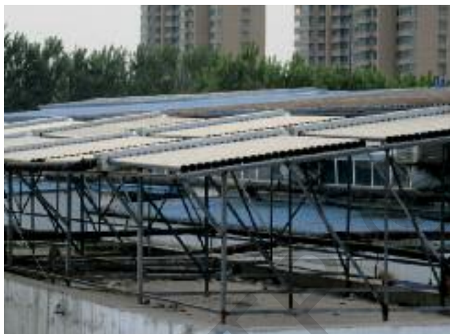
Solar powered water heaters in place on the roof of one of the tannery buildings. With an ability to heat the process water to 90°C in the summer and 50°C in the winter, the implementation of these heaters removed the need for a coal burning boiler that used 2,000kg of coal per day.
