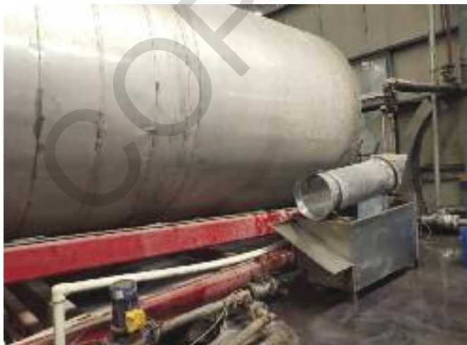
At the end of chrome tannage, the remaining float is passed through a perforated drum filter to remove solids. The resultant screened liquor is then held in the underground storage tank below the vessel for reuse with fresh chrome.
