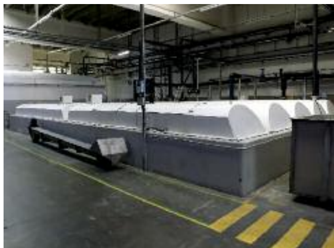
One of the two six-metre-deep 120m 3 wastewater holding tanks. The system was designed and installed by Italprogetti and occupies a space close to the far end wall of the tannery, closer to the main effluent treatment plant. There is very little smell in the whole area and the owners are rightfully proud of the investment.
