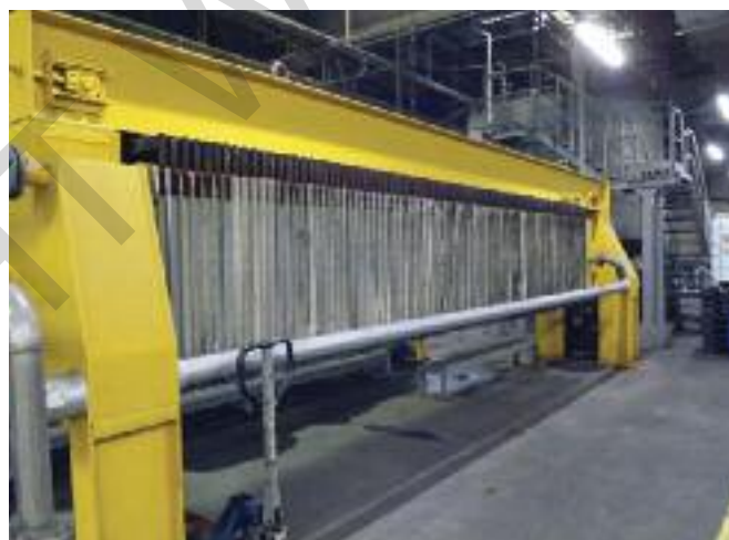
One of the four 100-plate filter presses used for precipitated chrome sludge cake production. The cake is hoppered into a macerator prior to acidification.
