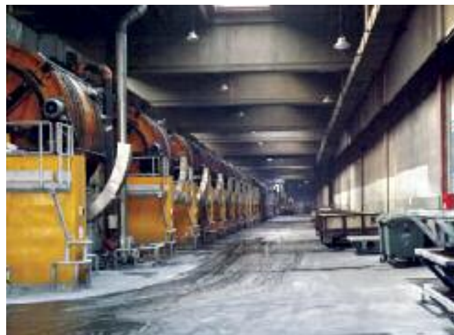
One of the banks of Hüni tanning drums all safely protected by optical 'magic eye' safety guards that isolate power, stopping the drum should personnel get too close to the drum whilst it is revolving.
