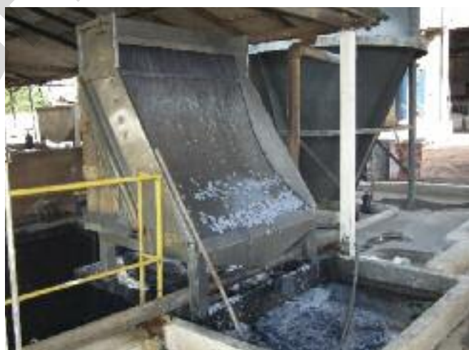
The effluent treatment plant at Sepiciler in Turkey. The greater the efficiency of the leather chemicals tanners use, the easier the burden on plants like this will be. CREDIT: WTP
