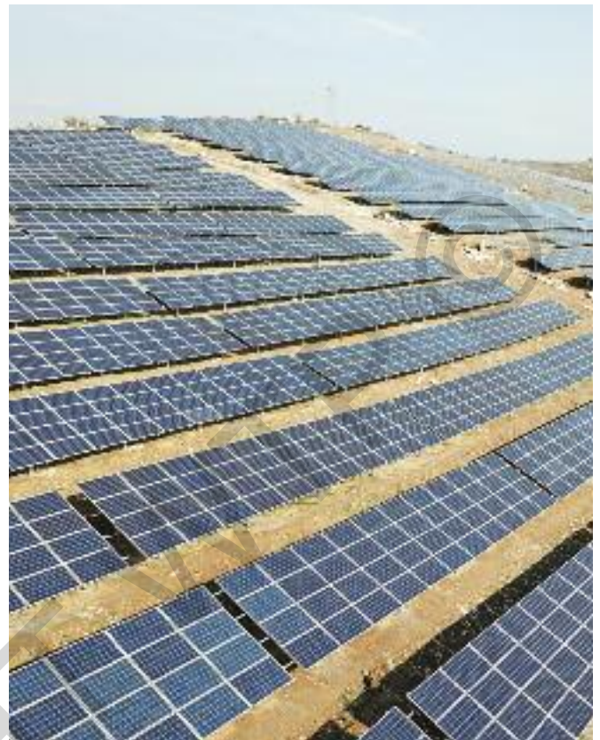
A new solar energy plant on land close to the tannery will deliver back to Turkey's power network six times the amount the tannery uses to make leather.
