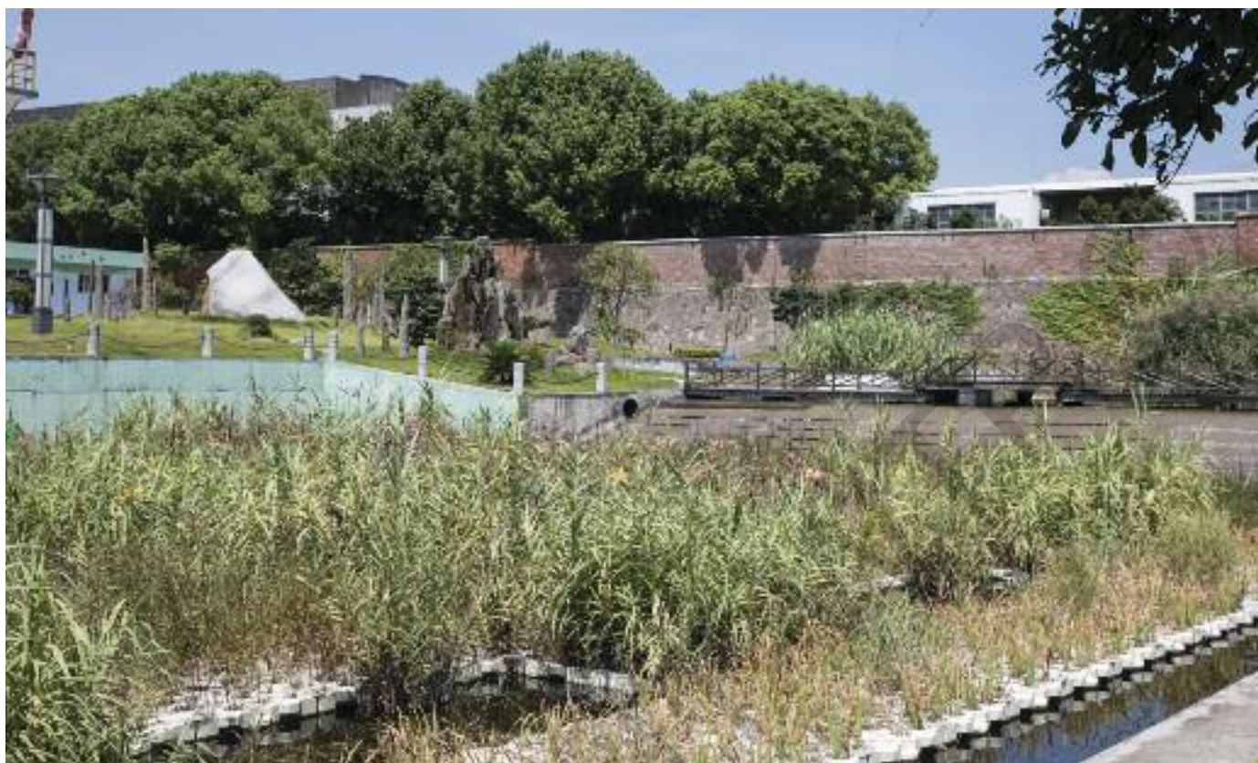
The effluent treatment plant at the Tongtianxing tannery in Zhejiang province. Environmental requirements are probably the main reason why the number of tanneries operating in China has dropped from 1,800 in 2011 to 600 now. CREDIT: TTX
