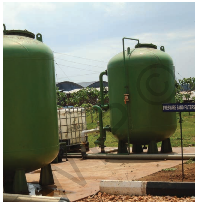
Pressure sand filters are in place to help LIU make the liquid effluent it discharges as clear as possible.
