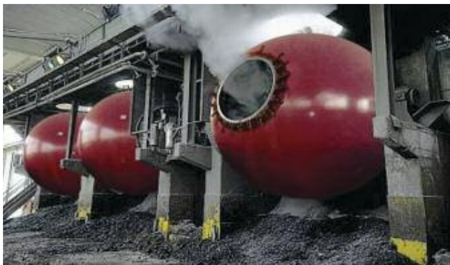
Thermal hydrolysis plant – Ilsa SpA, Arzignano (VI)
