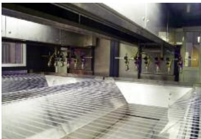
Internal view of cabin with two gun carrier drives. Spray guns and robots can be seen.
