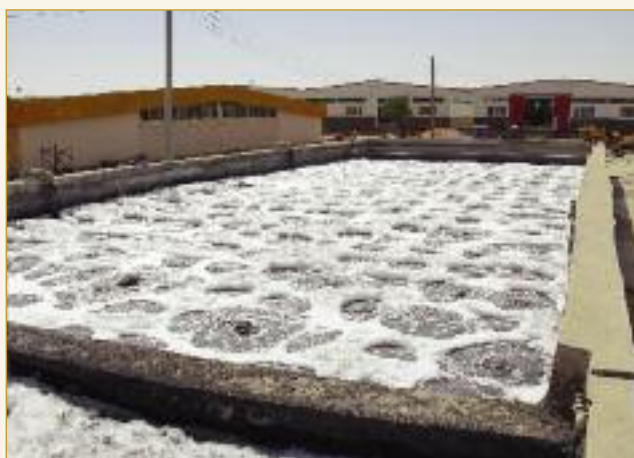
The effluent treatment plant has been upgraded with assistance from UNIDO. The capacity is greater than required at present, and can cope with the inevitable surges in input due to fluctuations in hide and skin availability.
