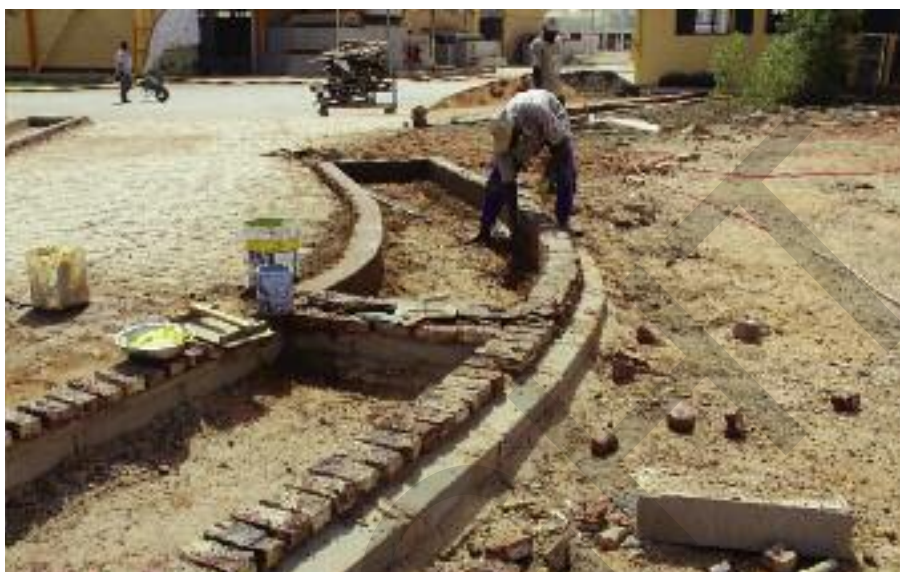
The original site was largely barren, but is now being landscaped with pathways with borders for flowers as shown in this area next to the effluent treatment plant.
