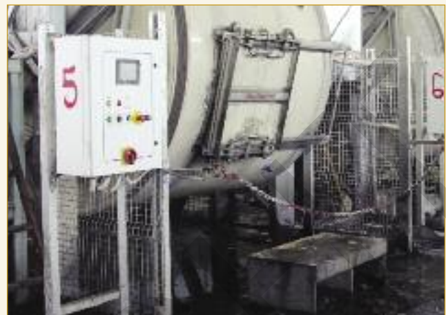
The dyeing department is being upgraded, and this shows the first pair of recently installed plastic drums that have now been brought into operation.
