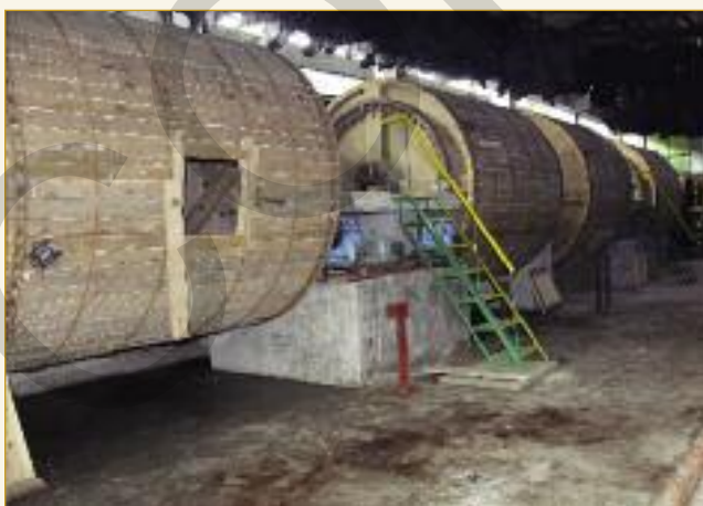
This row of drums is being installed by the tannery to create a new vegetable tanning department. Each vessel has a capacity of 4 tonnes input weight, and once in operation it will be possible to separate used vegetable tanning baths for reuse.
