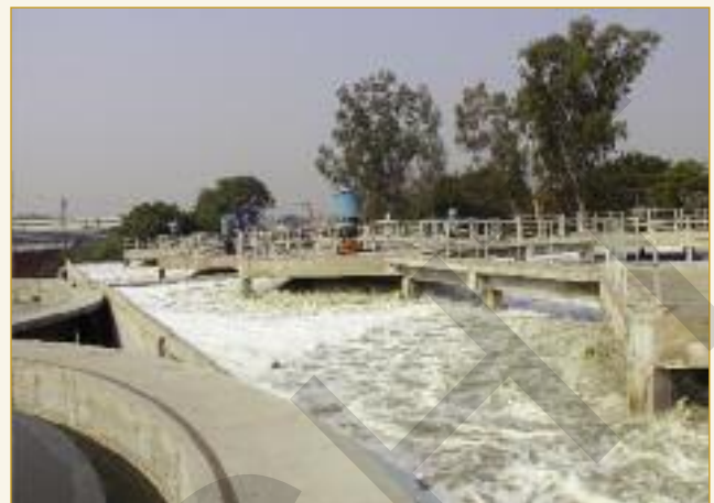
The effluent is finally treated by the CETP plant located less than 1km from the tannery. This effluent treatment plant does not chemically dose the effluent, but has extended the biological treatment to four days' retention time.
