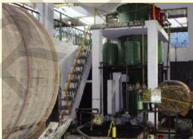
The chrome recovery plant uses magnesium oxide as the source of alkali for precipitation. The settled chrome sludge is discharged directly into the reaction vessel set below the settling vessel for the regeneration of chrome liquors.
