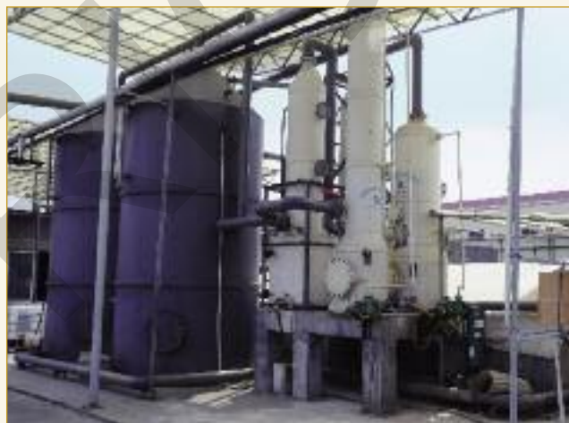
Sulfide containing wastewaters are acidified in the two sealed tanks to the left, and the evolved gas dissolved within the two columns to the right to regenerate sodium sulfide for use in liming/unhairing
