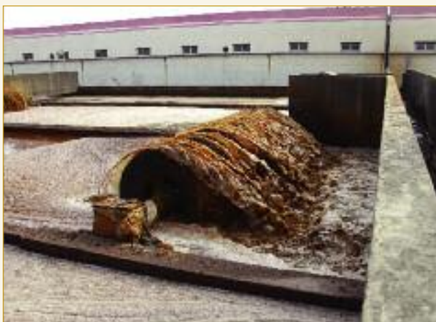
The Pasveer ditch has sufficient capacity to retain the effluent for one day for biological treatment. The image shows the wire brushes used for circulation of the effluent and the introduction of air into the system.
