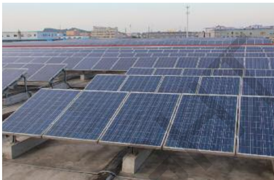
Solar panels cover around 50,000 square-metres of roof space at Dazhong Leather generating approximately 5 GWh of electrical power per annum. This makes an important contribution to the company's policy of saving money on energy while also contributing to cleaner air for the city of Haining.
