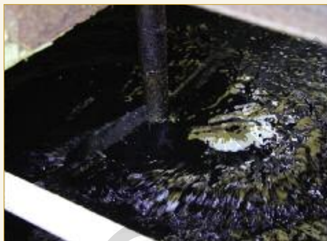
All of the chrome wastewaters are segregated. After precipitation, the chromium hydroxide is dried by filter press, and the cake dissolved in sulfuric acid as shown before pH adjustment.
