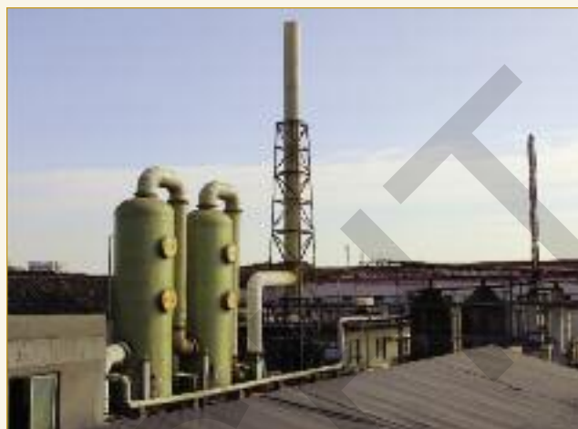
All parts of the effluent treatment plant where airborne odour can occur are covered with heavy-duty plastic covers. Air is continuously extracted and washed to remove these components using two scrubbing units before discharge to atmosphere.
