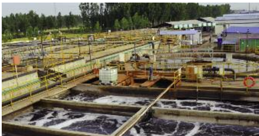
The new main effluent treatment plant at Meihua Leather Co.Ltd.
