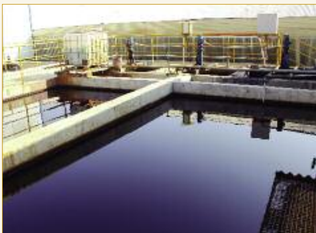
The discharged floats from dyeing, retanning and fatliquoring are treated separately in a dedicated wastewater plant. This is equipped with its own filter press to dewater the precipitates that are formed by chemical dosing.
