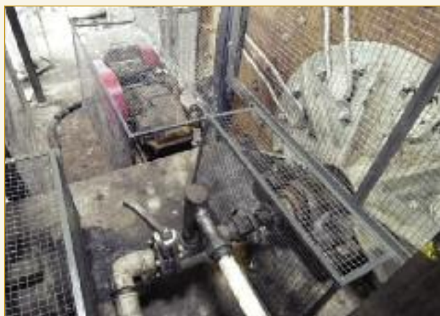
The guarding of the processing drums is extensive. Guarding of the front, rear and mezzanine service area has been extended to cover the sides of each vessel, the axles, motors and gearboxes, and belt and cog drives.
