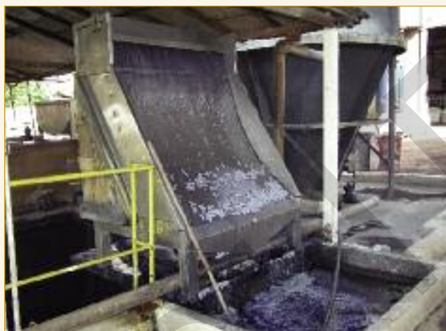
The used floats following chrome tannage are screened to remove solids on a wedge-wire screen. The filtered solution is then allowed to settle to remove residual fine suspended solids before reuse in subsequent tanning processes.
