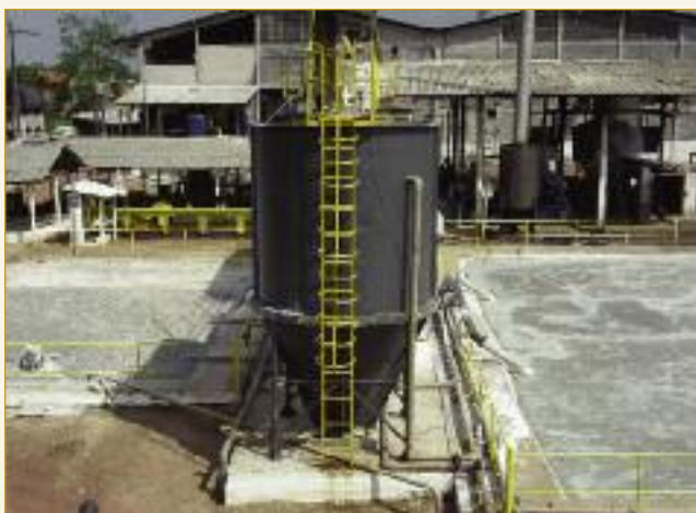
After mixing for balancing, equalisation and aeration (left), the effluent is chemically dosed and settled in a row of four reaction and settling vessels operating in series. This is followed by biological treatment (right), then secondary clarification.
