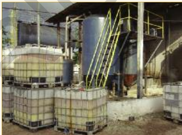
All of the fleshings are cooked in vitreous steel tanks to release fats and grease. This extract is decanted and stored in poly-crates before sale for soap and other products.
