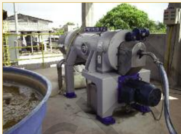
All of the solids from primary and secondary clarification are dewatered to approximately 25%. The centrifuge is mounted so that when the solids drop to the floor they can air-dry before being removed by bob-cat.
