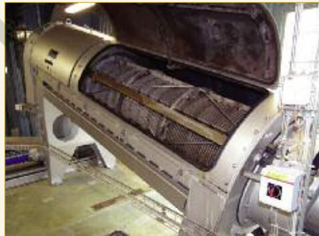
All of the settled solids from primary, secondary and tertiary clarification treatment are chemically dosed, then dewatered to around 28% solids in this huber screw press. Essentially a cylindrical bar screen filter, solids at the base and sides are compressed as they are slowly screwed towards the top of the inclined cylinder before discharge.
