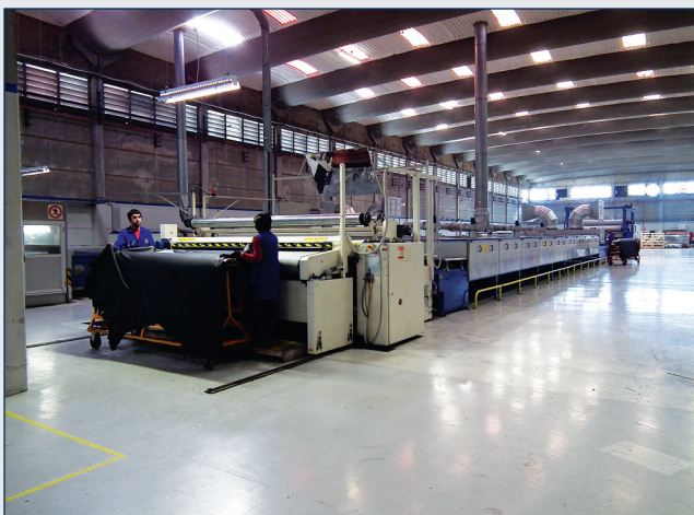
Pristine conditions are being used by leather manufacturers within finishing operations to minimise contamination. This includes control of temperature, relative humidity, and air filtration.
