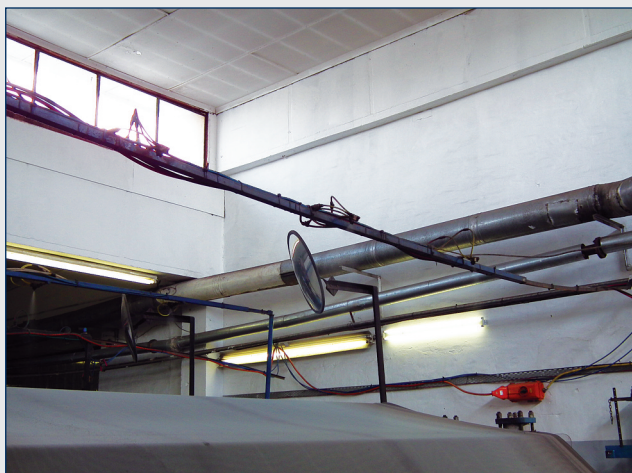
The relative humidity of air is being managed by spraying a mist of water as required into the air within appropriate departments.
