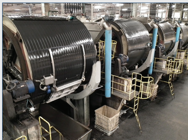
Separated and recovered solids are extracted from the screening arrangement and delivered into waste containers set at floor level.
