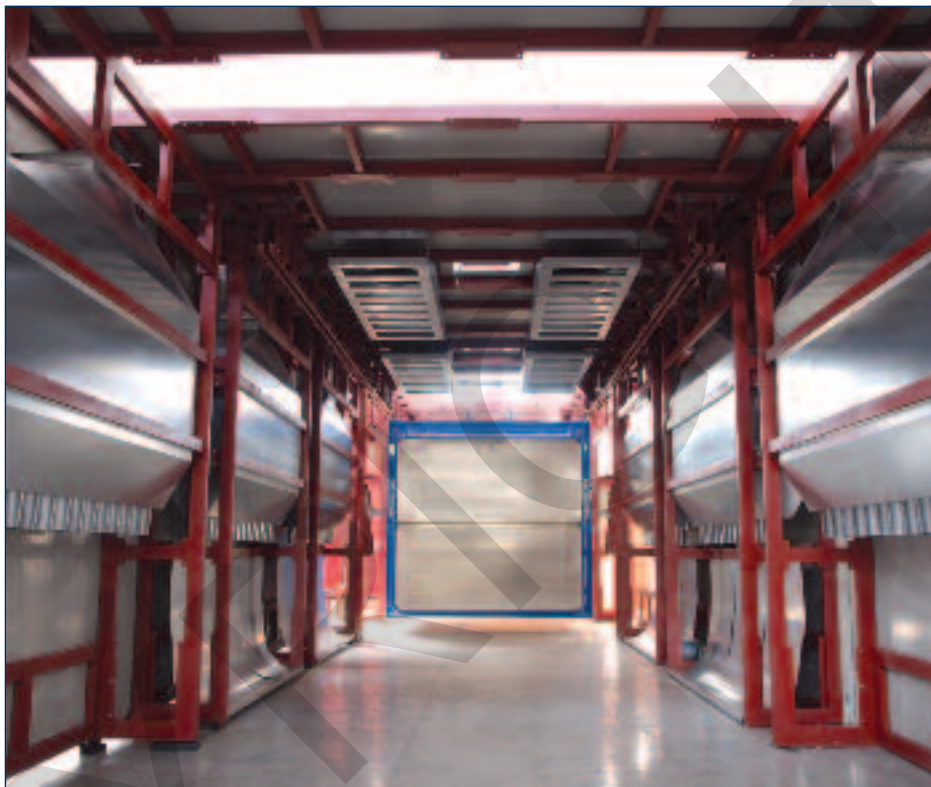
Inside view of cell rotaring conditioning toggle dryer.
