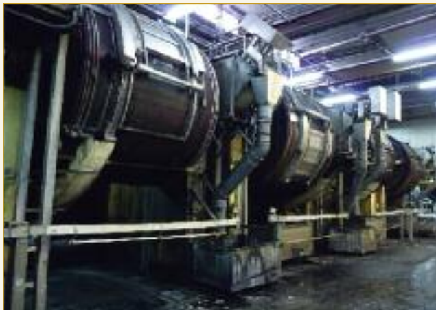
Four 3 x 3.5m Olcina dyeing drums. All of the eight are equipped for recirculation and continuous removal of solids from the dye bath.
