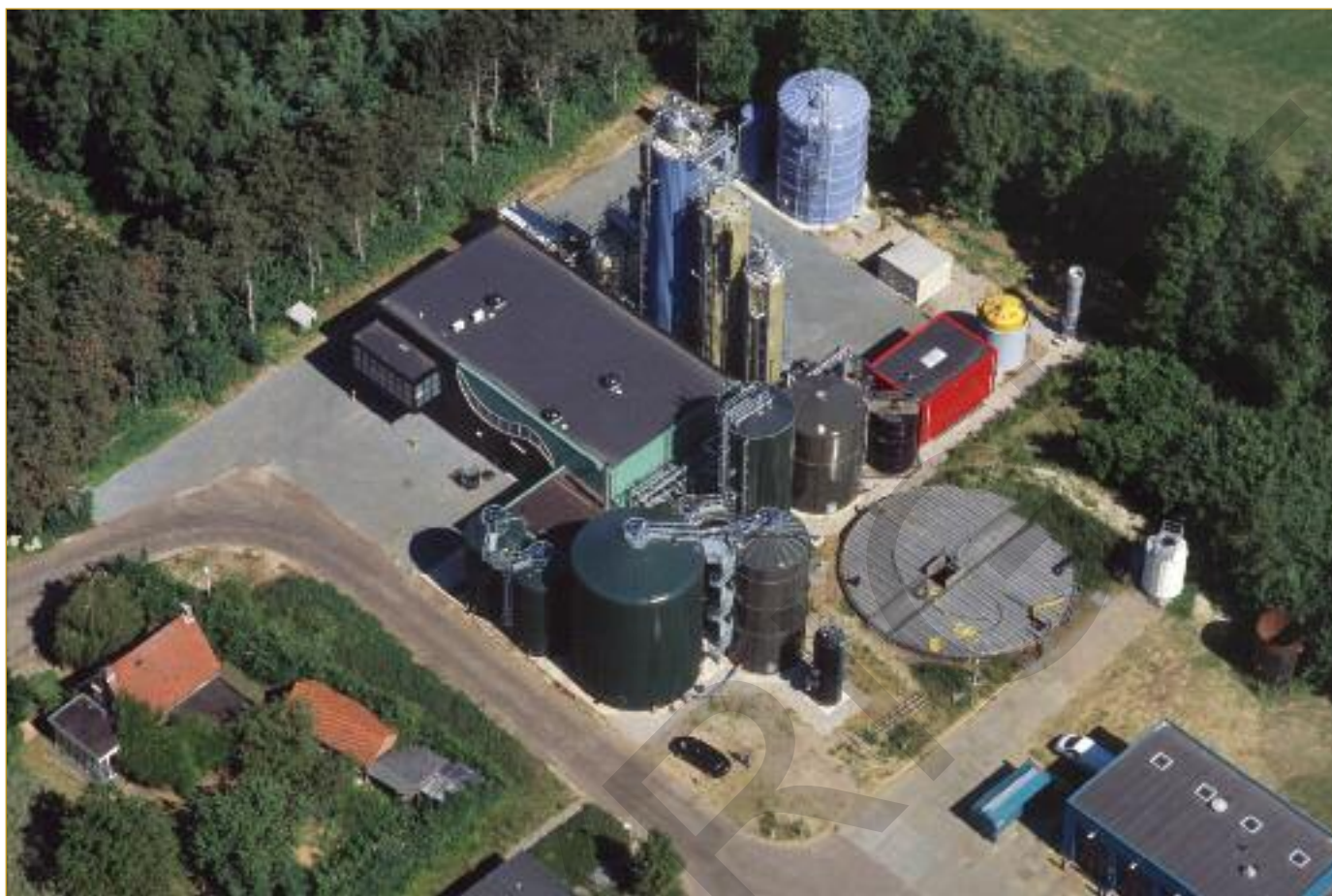
Overview of the tannery effluent treatment plant. This is situated near to the municipal treatment plant, and both are located on the same site in open countryside. CREDIT: HULSHOF
