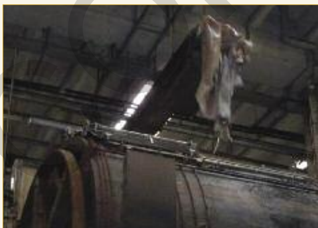
The conveyor line for delivery to the tanning drums rises above the service mezzanine for the tanning drums. The system then delivers the goods to the selected tanning drum.
