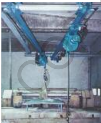
Danese loading gantry transferring skins to a fleshing machine.
