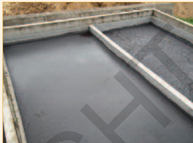
All of the chromium-containing wastewaters are precipitated with lime, and the settled sludges then dried using two sand filters. The supernatant is delivered to the balancing tank.
