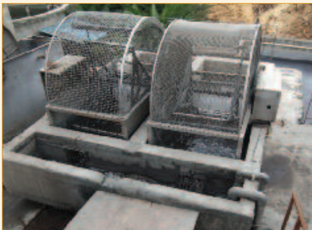
All of the effluent is screened through this pair of self-cleaning stainless steel screens that operate in parallel. Wastewaters are collected in a small collection sump after screening, then directed for either oxidation of sulfides or for general balancing.
