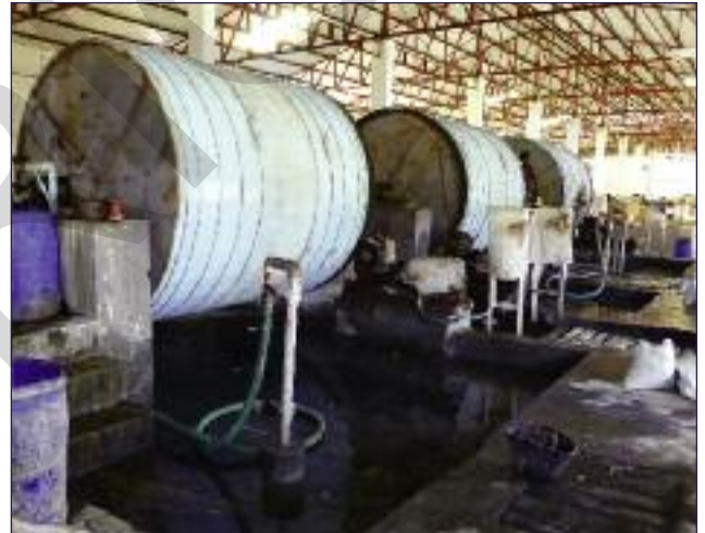
The tannery has three drums used for chrome tanning and it is intended to install a chrome recovery plant.
