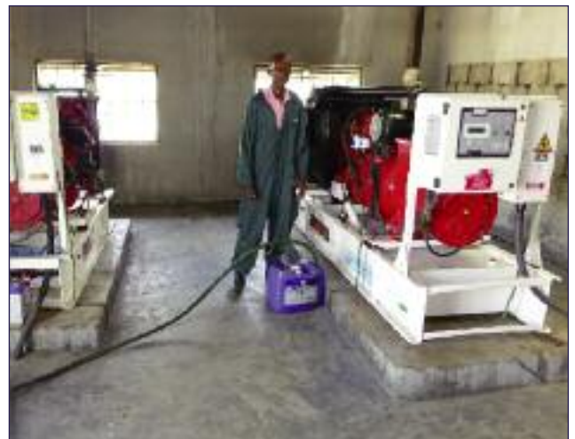
There is no electrical supply to the tannery, so power is provided by the on-site generator.
