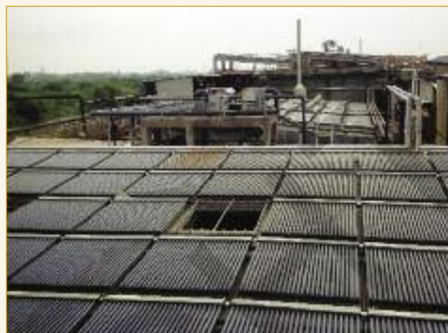
The areas for primary and secondary effluent treatment are roofed to reduce odour. In addition, these areas are fully covered with solar panels through which the effluent is circulated to raise the temperature by 10°C, and thus improve the efficiency of the biological treatment.
