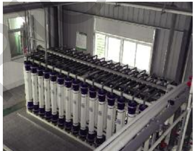
An ultra-filtration unit with treated effluent going through final preparation for reverse osmosis.
