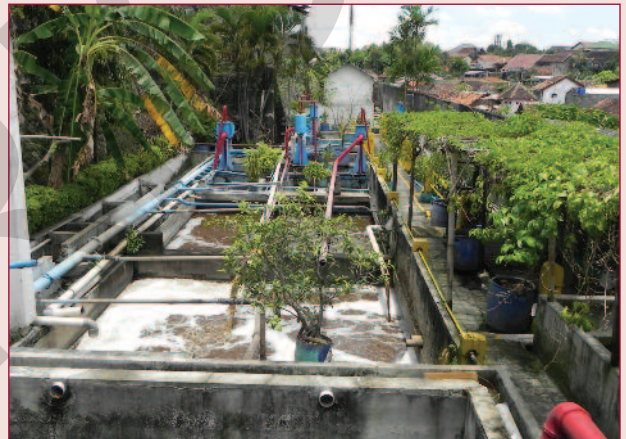
PT Budi Makmur tannery is located in a residential area. Not only are the wastewaters treated to a high standard before discharge from the site, but the whole of the effluent plant and the walkways have been softened by extensive "greening".
