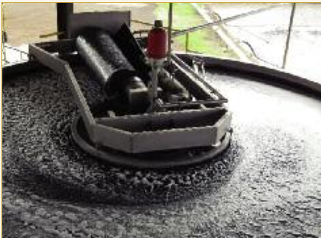
Within effluent treatment, after chemical dosing, solids are removed from the surface of flotation units. Rotating scoops, as shown, are used to remove these solids before dewatering by centrifuge.
