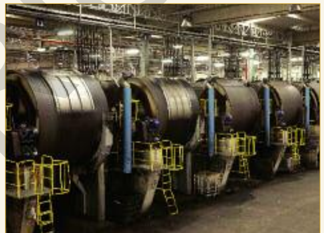
Part of the line of seven Hüni deep-shelf drums in the dyeing department. Seven conventional wooden drums of 4.0 x 4.0m by Michelin are placed on the opposite side of the service mezzanine.
