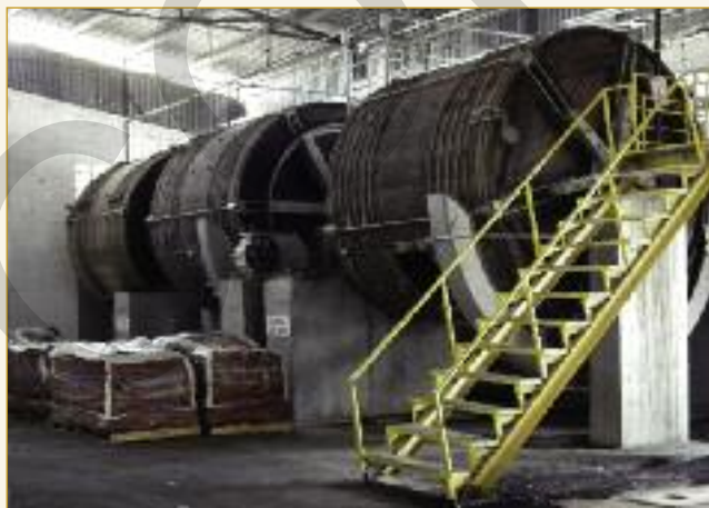
Three of the six drums originally used for soaking, liming and tanning. Together with a fleshing machine and a lime splitting machine this plant is being held in mothball following the extensive flooding experienced by the tannery.
