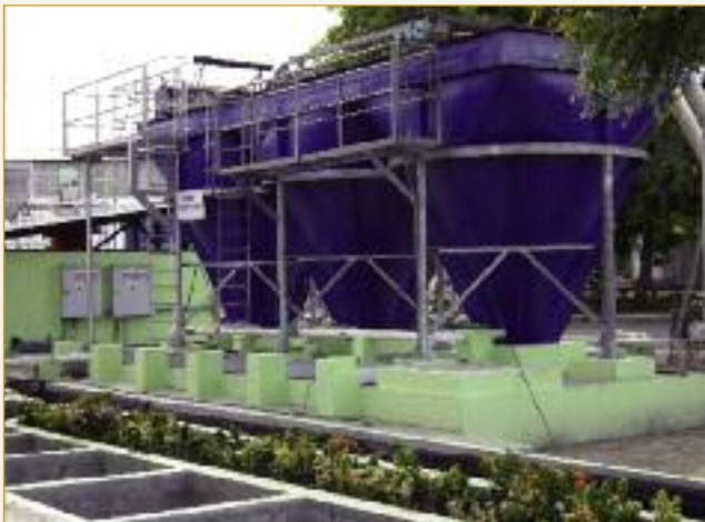
The three settling cones where the primary effluent is first subjected to flotation and settling. Gross solids are first removed using a self-cleaning screen on top of the plant. The effluent treatment area is bunded, and flower beds have been created within the area.
