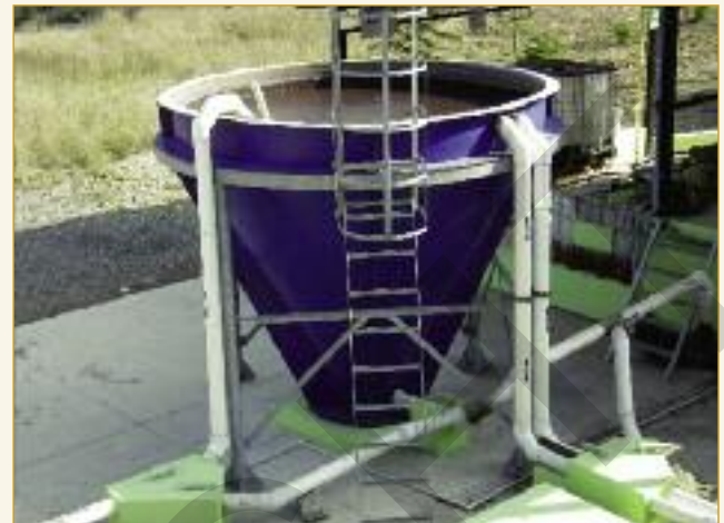
The sludge thickening tank where sludge from the initial flotation and settling, and settled sludge's following chemical dosing are blended to release water. This concentrates the sludge before offer to the belt press for dewatering.
