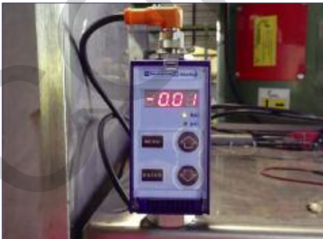
Depressurisation system controller.
