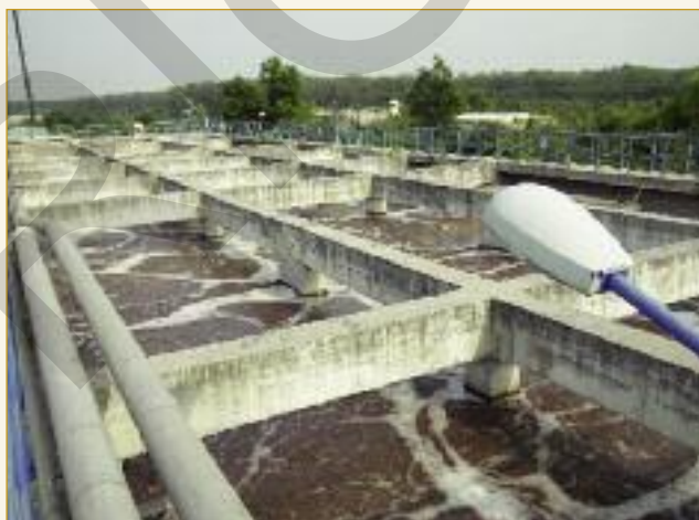
Conventional activated sludge treatment is used for secondary treatment, but settling of the biomass is assisted by dosing the effluent at the point of outflow with aluminium salts and polyelectrolyte.
