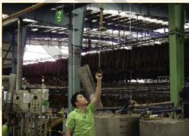
Because of the dangers of manually adding chemicals to feed-containers in the dyeing department – especially acids used for fixation – there are easily operated overhead showers fitted over each of the 14 feed-containers to drench the operative in the event of contamination.
