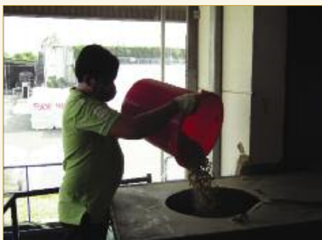
At the present wood chippings are fed manually into each of the two biomass boilers that are now providing 35% of the energy use for this plant. The system is being modified to automatic feed.
