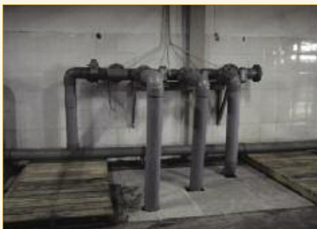
Each drum has an option to segregate used neutralising, retannage-black dyeing, and fatliquoring baths for recycling in following loads. The remaining used floats are discharged directly to the effluent treatment plant.
