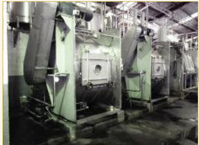
The two Unimat dyeing machines are heavily used as very close control can be maintained during the dyeing process. The Haigspiel processor is shown to the right.
