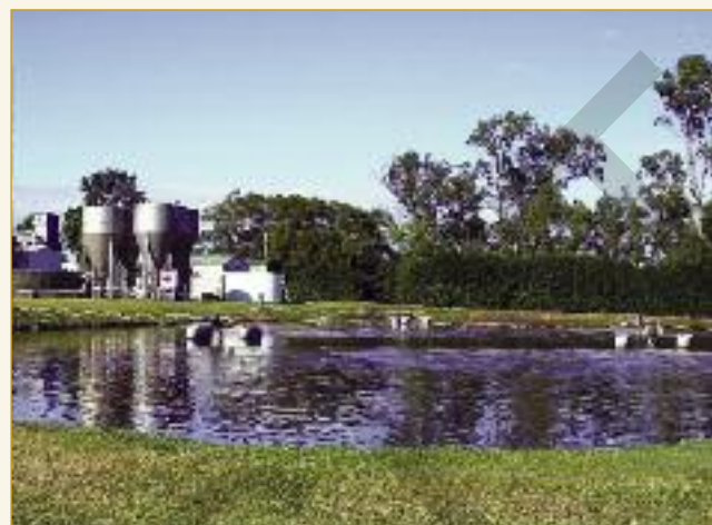
After primary treatment and settling using two of the settling tanks shown, the effluent is subjected to biological treatment in two lagoons operating in series. Aeration is provided by cavitation aerators set on floating pontoons.
