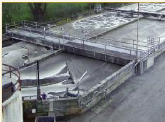
This raceway is being used for separation of residual fine solids after conventional secondary effluent treatment. A small volume of air is introduced to create a scum, and this is directed (low left) towards a belt mesh that lifts the scum and entrapped solids from the surface.
