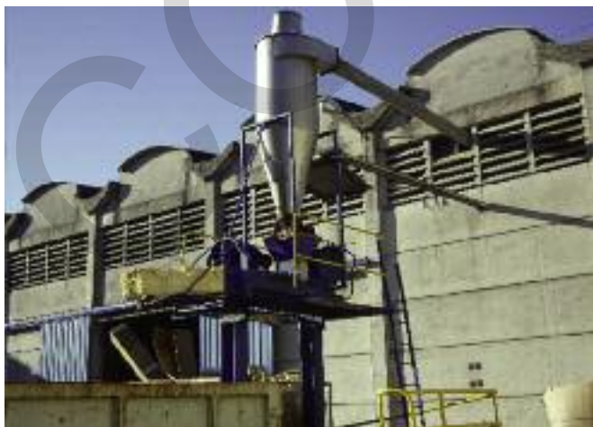
All of the shaving dust is blown from the shaving operation to an elevated cyclone set outside the building for compression before deposit into a hopper.
