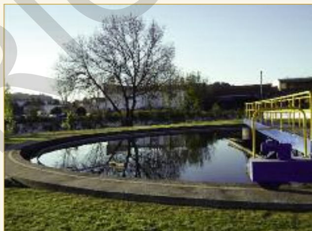
The common effluent treatment plant (CETP) receives pre-treated wastewaters from around 50 tanneries in the Alcanena cluster. The image shows one of the pair of secondary clarifying units.
