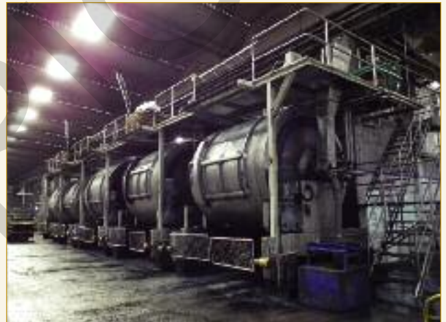
Dyeing, retanning/lubrication is performed in Dose tri-compartment drums of equal size. The feed mezzanine is constructed of steel lattice and extends over the top of these vessels. Additions are by chute through feed hoppers or through the floor into the open drum.
