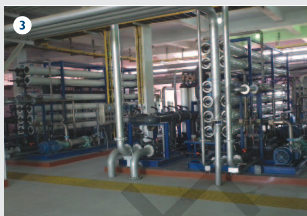
Reverse osmosis treatment in three units as shown above provides approximately 75% permeate as high quality water suitable for processing leather.
