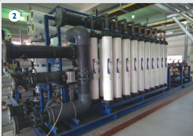
After extended tertiary effluent treatment, all remaining suspended solids are removed by ultra filtration.
