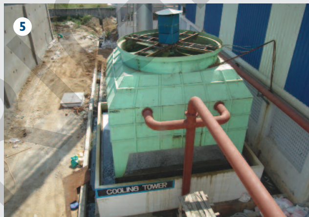
The evaporated water vapour is condensed and cooled in the cooling tower, then mixed with the recovered permeate from RO in a holding tank.
