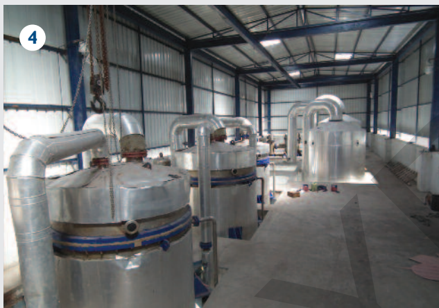
The remaining concentrate from reverse osmosis is evaporated to dryness in a series of seven stainless steel evaporators (tops of the units shown in the image above).
