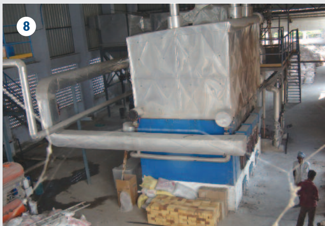
Two CEPT employees standing near the wood and biomass steam generating plant that provides energy for the evaporation of concentrate.
