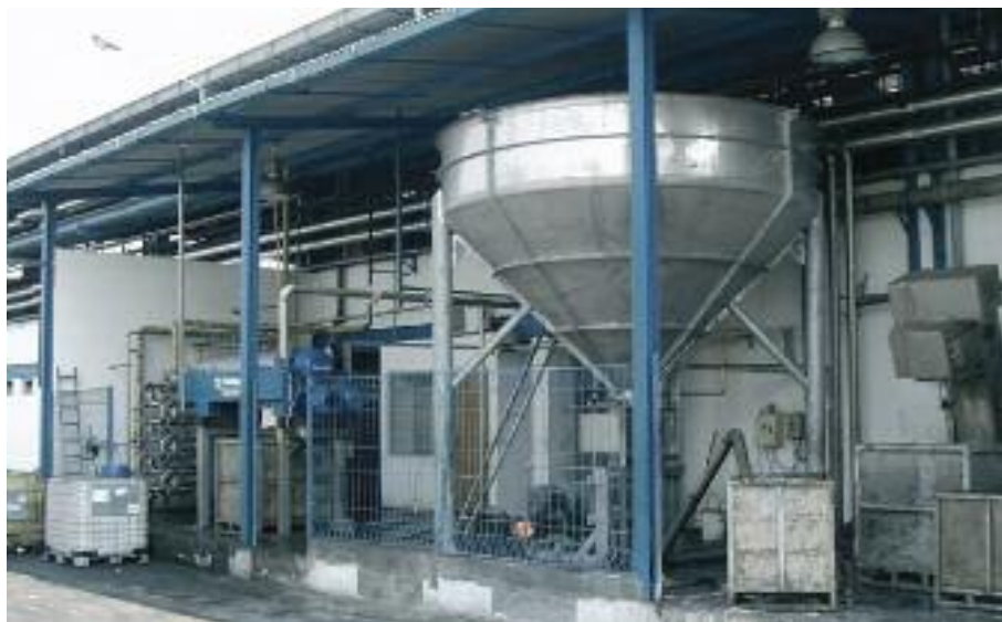
The equipment at the Indonesian tannery that Ecco is using to convert fleshings into fuel.
