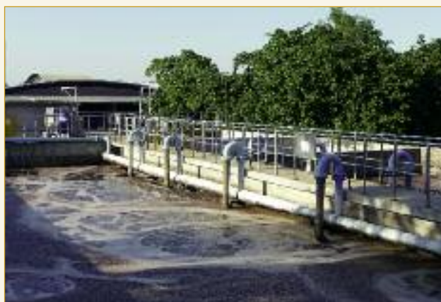
Part of the activated sludge treatment process within the tannery effluent treatment plant. The site was originally a cashew nut farm, and many mature trees have been retained around the site.
