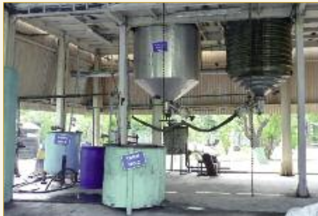
Part of the plant used to concentrate the hydrolysate recovered from shavings. Overspray from finishing is used with hydrolysate and binders to manufacture paint, as can be seen in the background.
