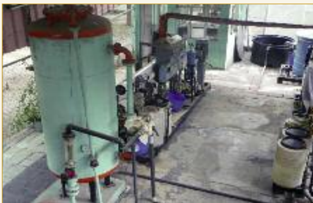
Photograph shows filter columns used to remove colour from treated effluent, and part of the reverse osmosis plant.
