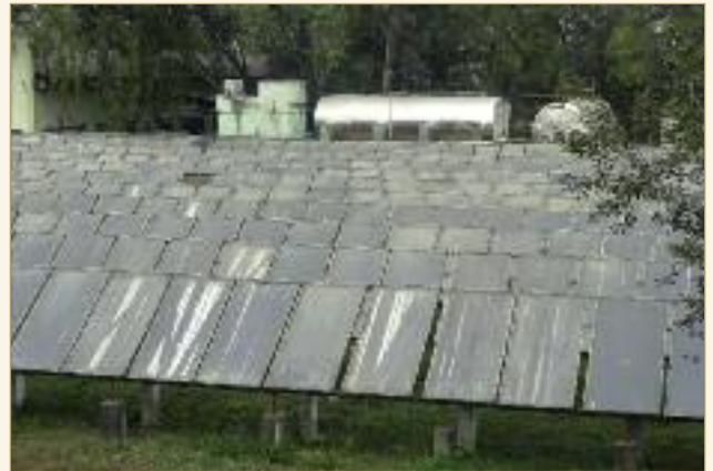
Each day, approximately 50m 3 the water from the reverse osmosis units preheated to 80°C using this array of solar panels, then used as feed water for the steam generation plant.
