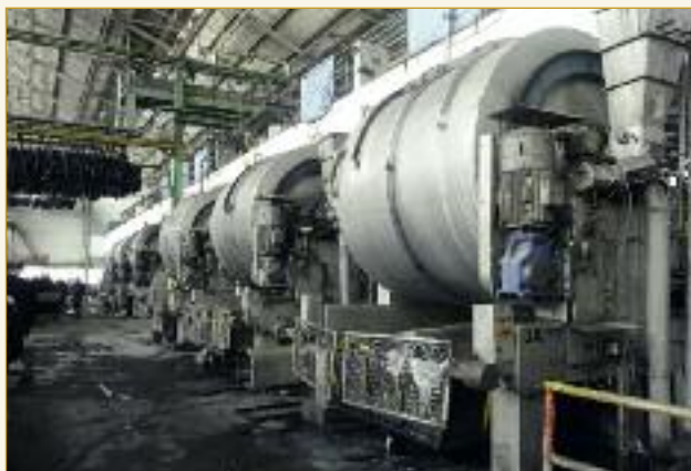
Part of the retanning/dyeing department showing a row of stainless steel Dose drums.
