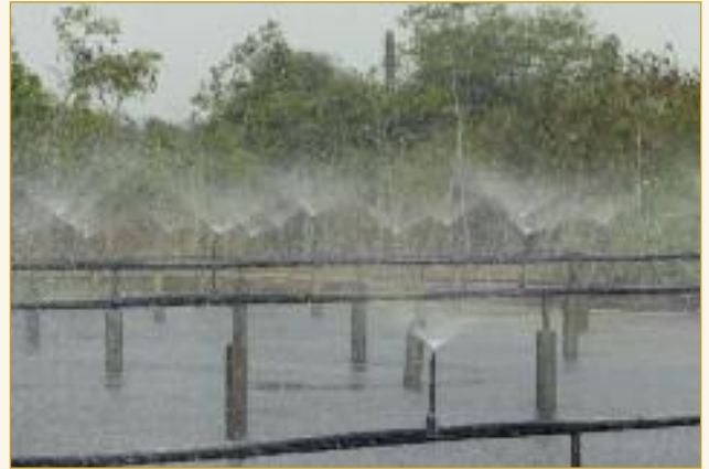
Part of the spray evaporation plant. Approximately 50m 3 of concentrate from reverse osmosis are evaporated to dryness each day. No effluent is discharged from the site and the dry solids are disposed to a government approved facility.
