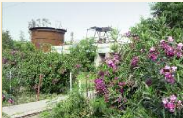
Trees and shrubs are used extensively within the area of effluent treatment plant. The vessel in the background is for anaerobic effluent treatment and the production of bio-gas for energy.
