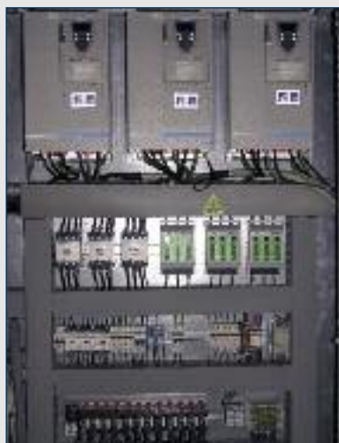
Inverter Controls of Exhaust Fans
