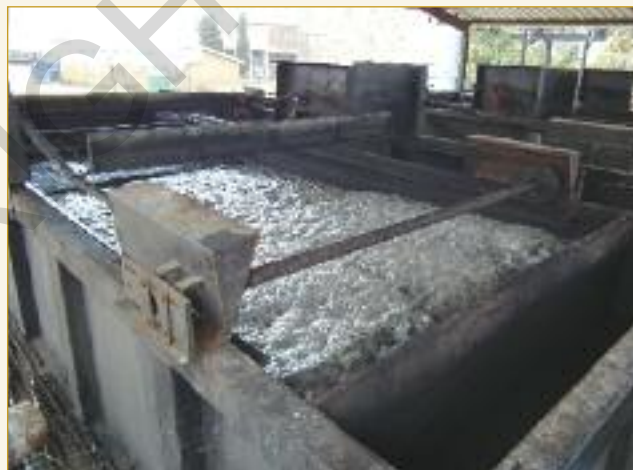
Precipitates and fine solids are held at a foam mat on the surface of the effluent by fine bubbles introduced into the base of a series of three air diffusion units as part of effluent treatment. This surface scum is automatically scraped from the surface, and then delivered to drying beds for dewatering.
