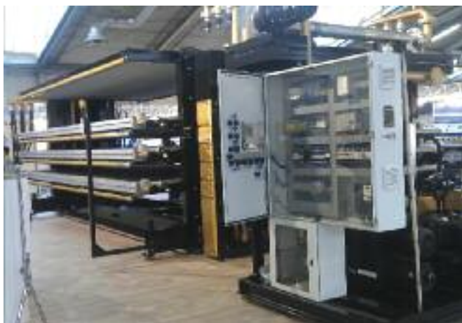
A multiple platen Turato vacuum dryer. Control panel is shown at the front with door open, electric motors seen directly behind the panel, drive the vacuum and recirculation pumps.
