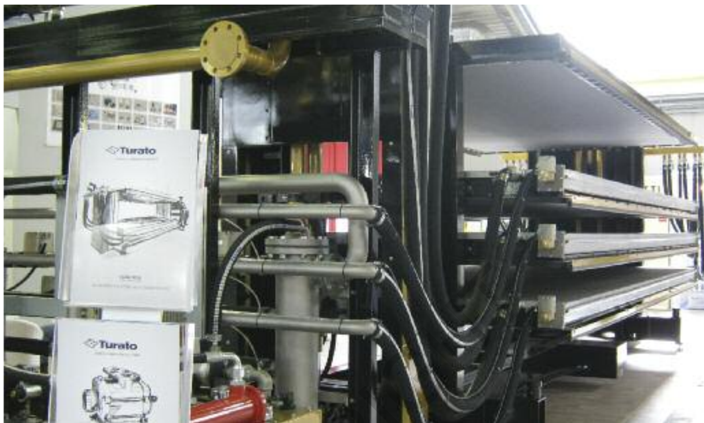
Large vacuum and recirculating pipework to platens and heads of a multiple platen machine.
