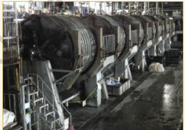
These six drums are used for soaking back all of the wet blue leathers. A wide mezzanine runs along the back of these vessels enabling easy movement of batches of leather for loading purposes.
