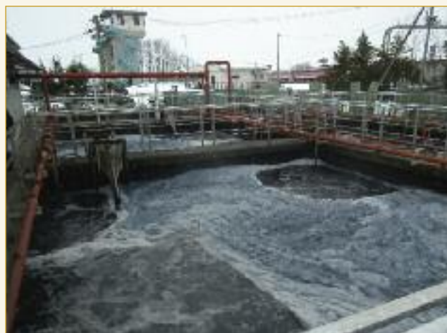
This photo shows part of the activated sludge treatment system. This comprises seven separate sections and this treatment follows chemical dosing with aluminium salts. The finally treated effluent is of a sufficiently high standard that it is discharged to the nearby canal.
