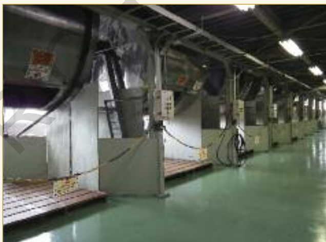
These stainless steel milling drums are set next to the finishing department and were manufactured in Japan.
