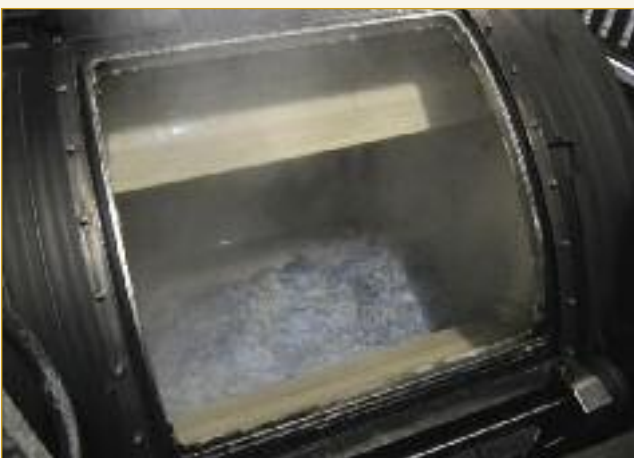
Three new polypropylene drums fitted with four deep shelves have recently been installed. These are used exclusively for automotive production.
