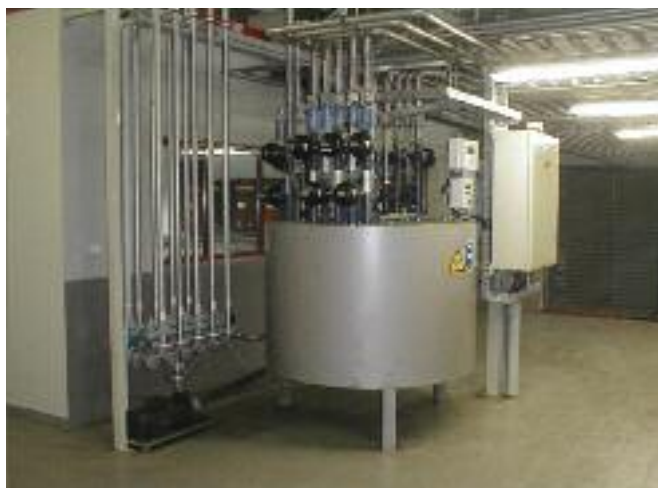
Prodromix mixing and dosing system with manifold scale tank and valve control housing.
